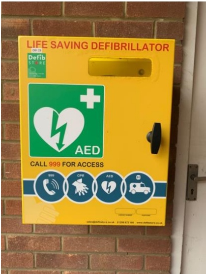
Community Centre – Defibrillator Cabinet
