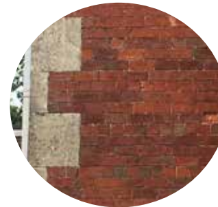
Stone quoins dress the corners of many buildings of different ages across the Parish
